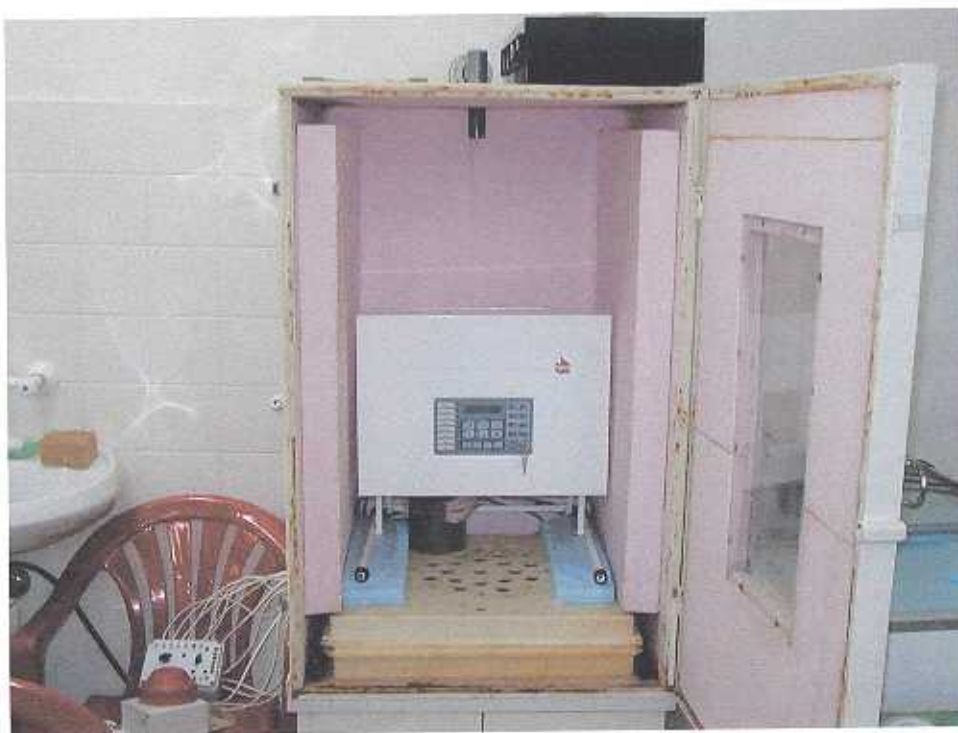
Photo 3: Humidity Chamber with Fire Control Panel FS 5100
