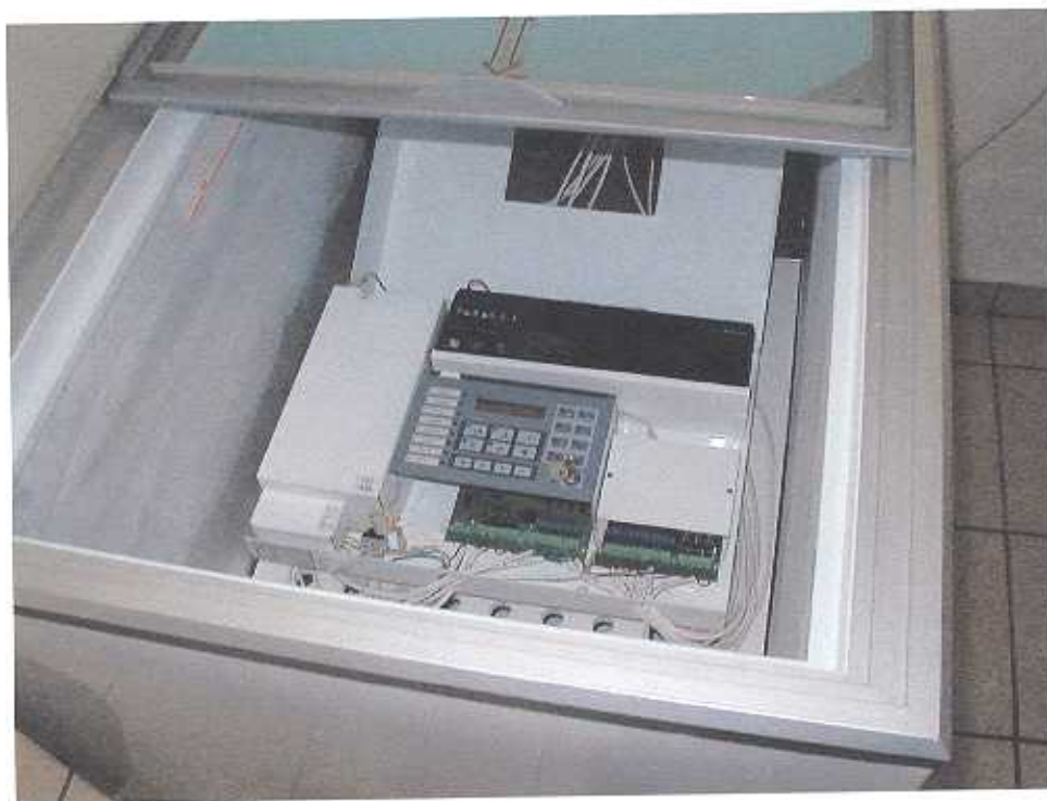
Photo 1: Cold Chamber with Fire Control Panel FS 5100
